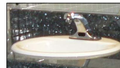
Water Efficient Sink Fixtures
